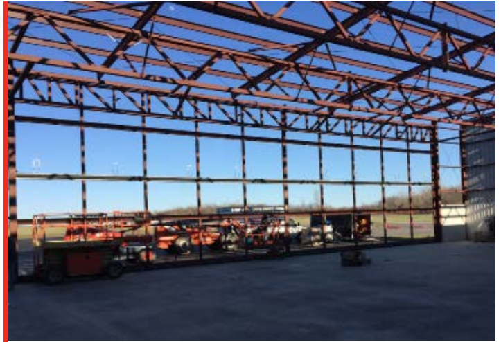
PROGRESS PHOTO OF NEW AIRPORT HANGAR AT LEWIS A. JACKSON AIRPORT -PHOTO COURTESY OF GENE TARTELL
