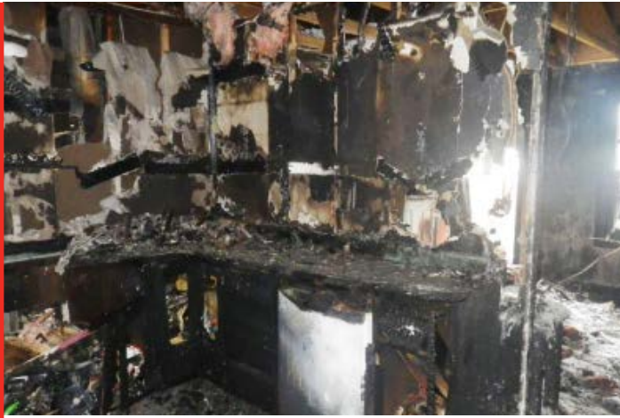
PHOTO OF ADAMS RESIDENCE AFTER FIRE LOSS -PHOTO COURTESY OF DAVE WILSON
