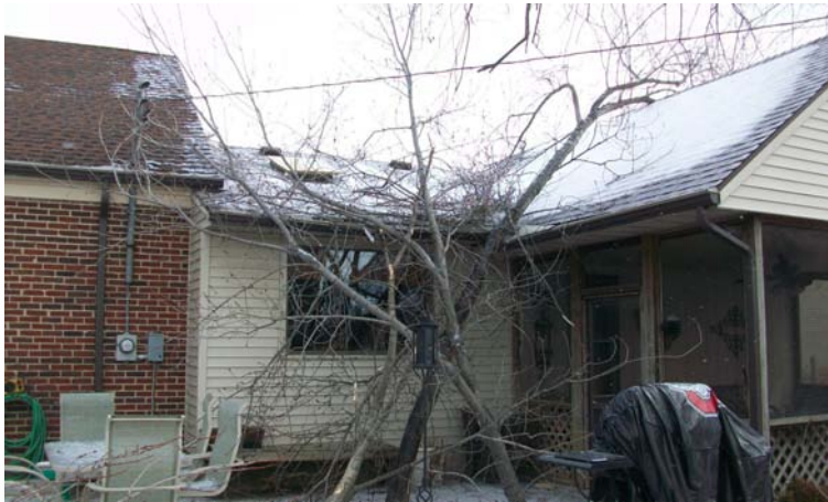
Example of Ice Damage at the Wilson Residence in Kettering— Photo courtesy of Troy Rosenberg
